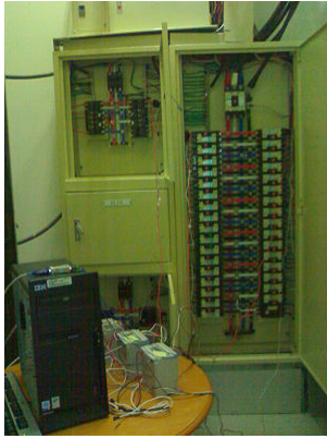
Figure 3. PA-310, electric panel and server
